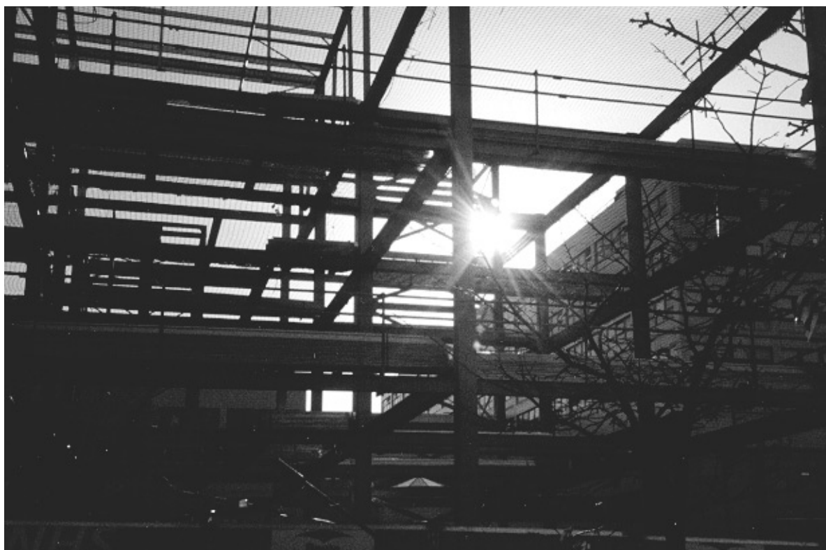
Up go the girders: and with PFI, up go the profits for each new hospital – replacing NHS assets with private
